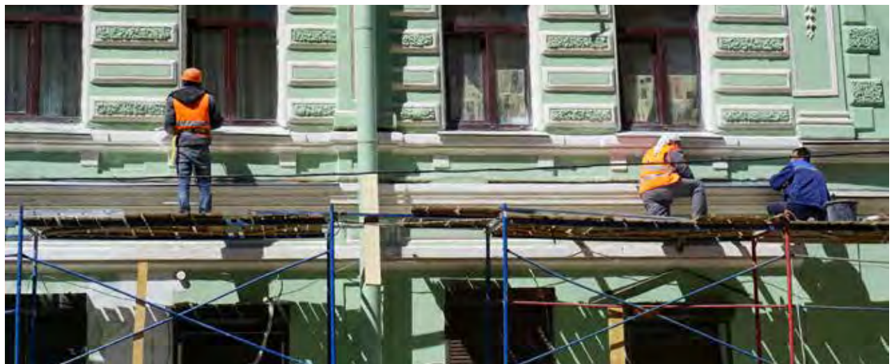
An example of downtown facades in need of renovation.
